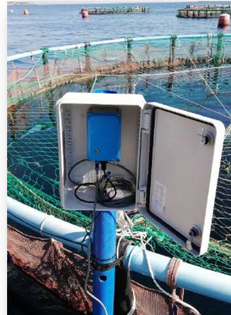
WINGS Smart Gateway installed in the site
